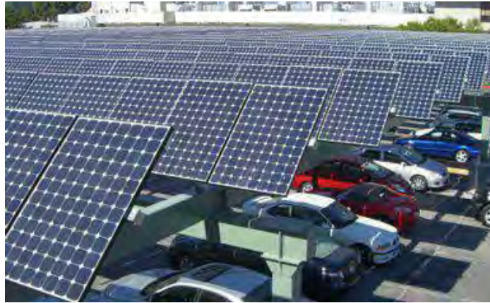
Figure 30: Solar Over Parking
