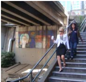
Stairways and paths to the water are unattractive and take visitors along and under highway structures.
