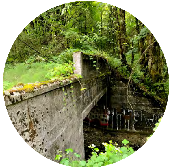
1. The old Sunset Highway bridge crosses over a creek. Grooves left in the bridge indicate cables were likely carts transporting carts of logs.
