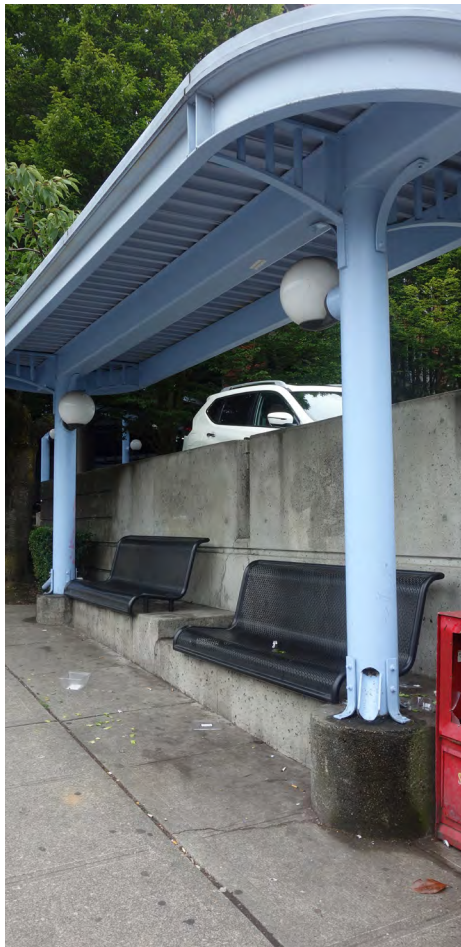
This bus stop seating area is clearly public and provides protection from rain and sun, but is not necessarily inviting.
