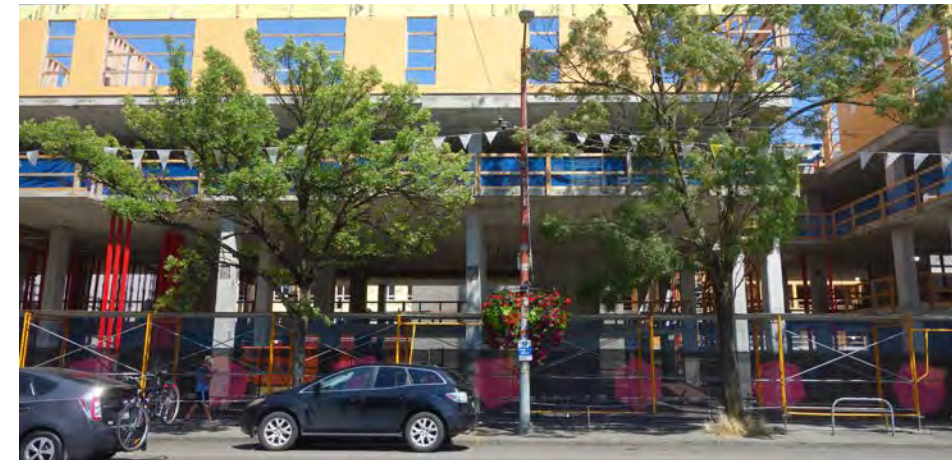
Buildings under construction in the area of the Capitol Hill light rail station will redefine the pedestrian experience of these block faces, which were not rated for frontage attractiveness.
